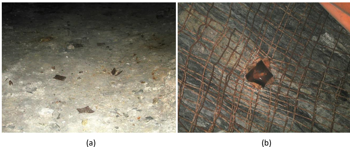
Figure 2 Highly loaded primary support. (a) Bolt plates on floor; (b) Highly deformed plate
