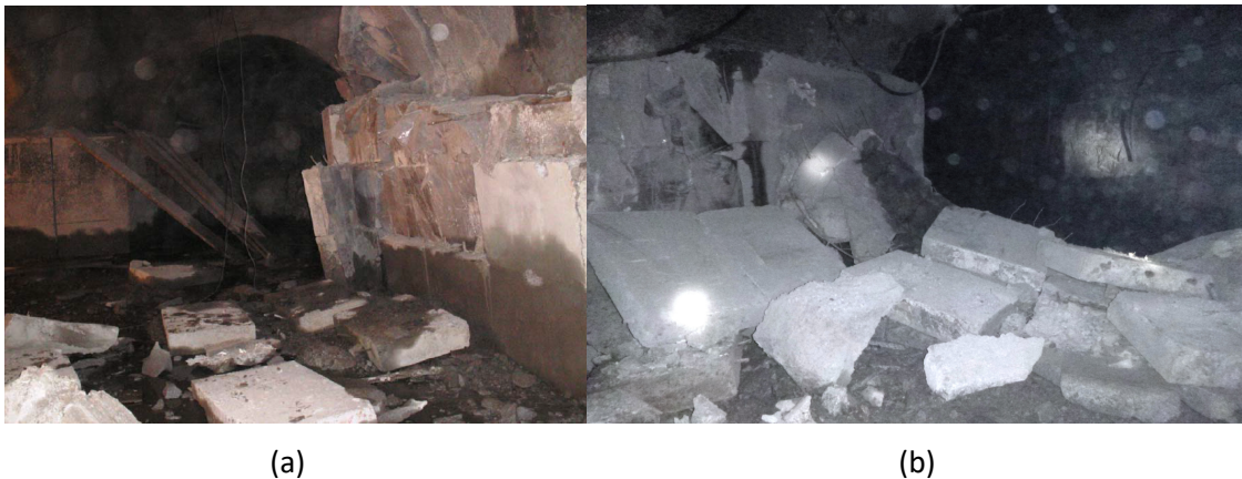
Figure 4 Concrete mass ejection in Pilar Norte El Teniente. (a) January 2010; (b) February 2017
