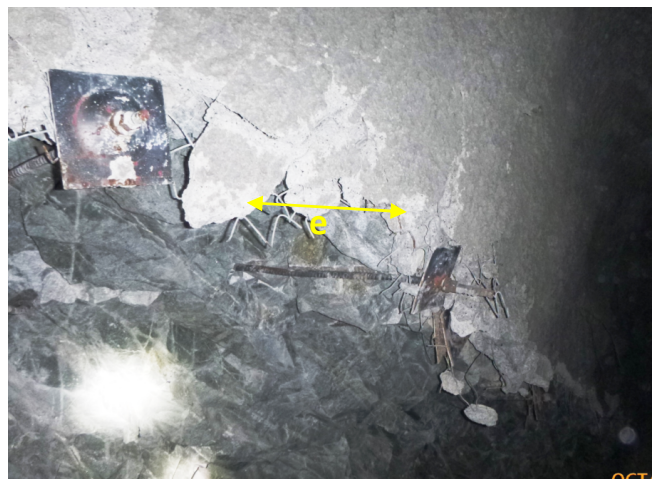
Figure 5 Ground thickness of damage
