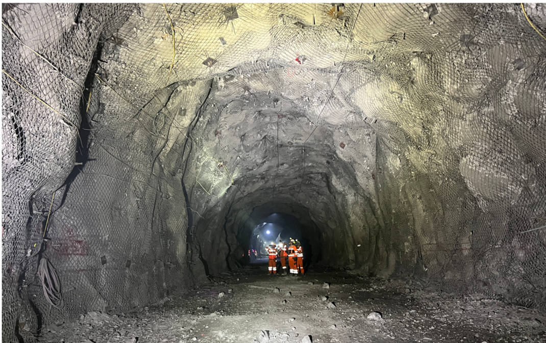
Figure 4 Photo showing the damage at the Tunnel Correa Interior Mina after a large seismic event
