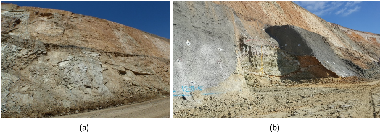
Figure 1 (a) Bench face conditions; (b) Bench mined back with fibrecrete applied to face and spiling bars installed
