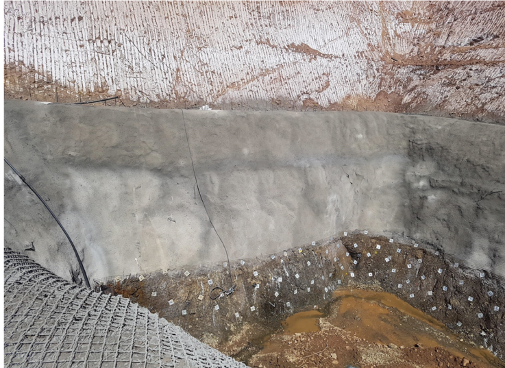
Figure 4 Portal face during excavation of the box cut with progressive installation of surface support and reinforcement
