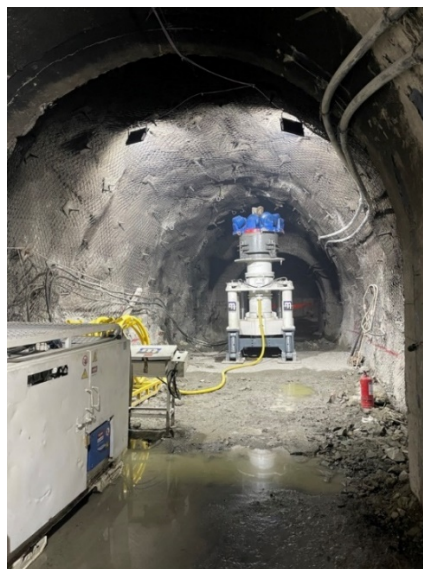
Figure 6 Blind hole machine installed and waiting to start shaft reaming, Andes Norte, El Teniente
