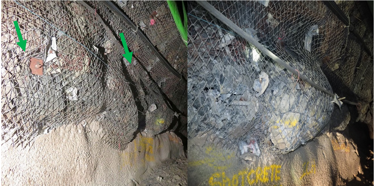
Figure 19 Examples of excessive deformation and bagging
