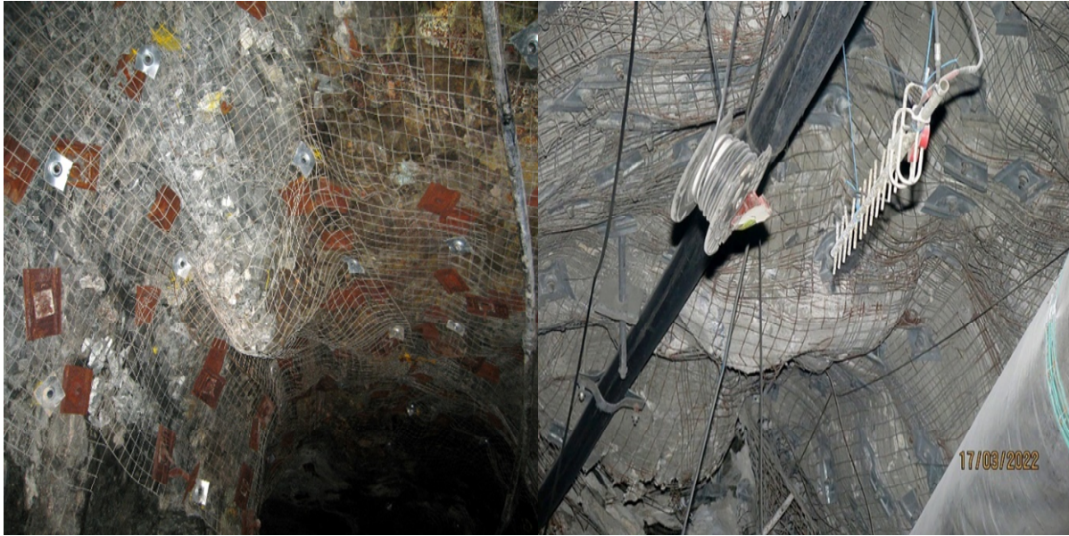
Figure 21 Examples of localised mesh bulking/nesting
