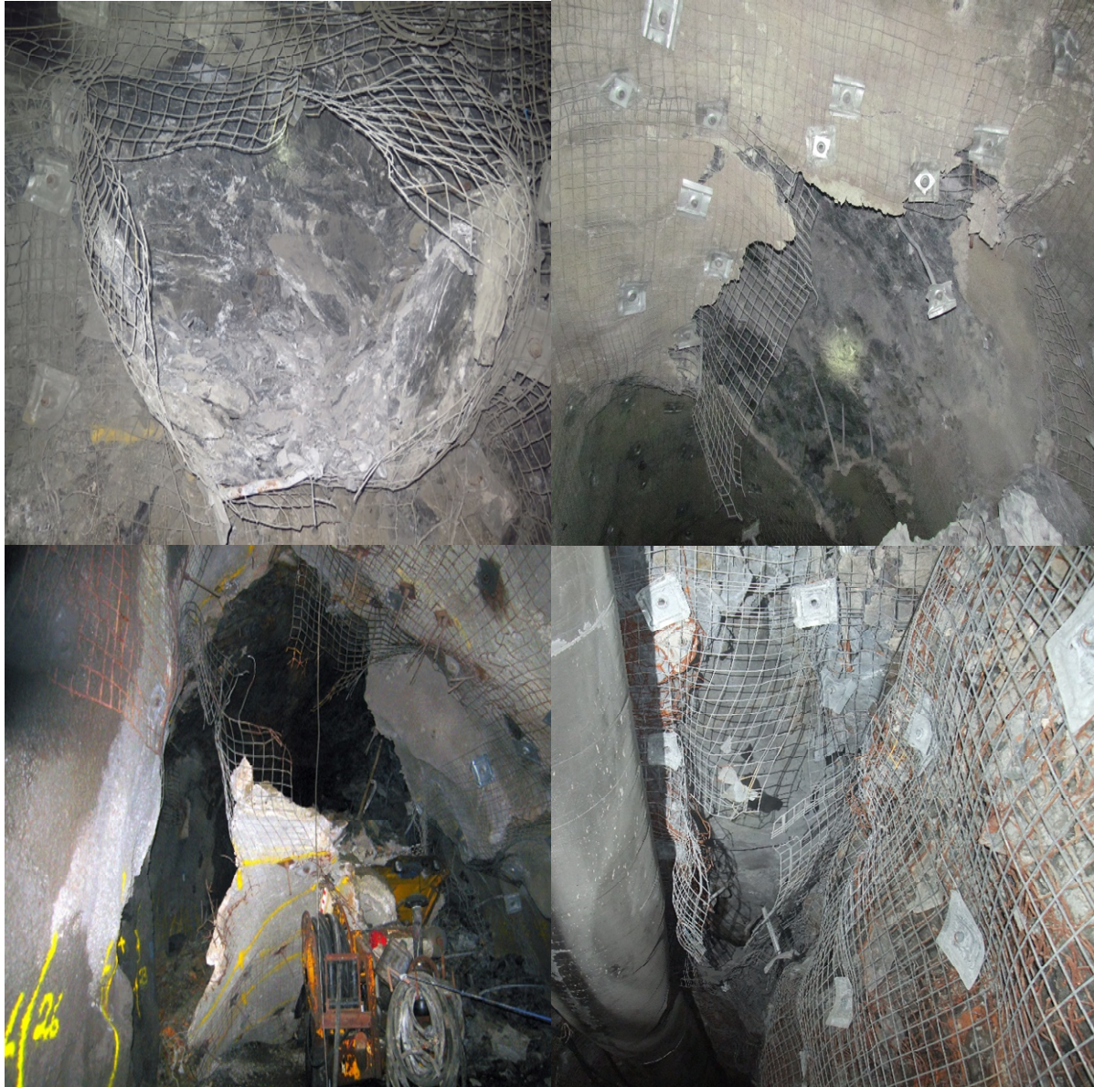
Figure 16 Examples of mesh tearing at the bolt–mesh interface
