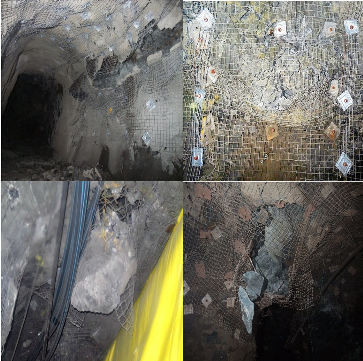
Figure 18 Examples of mesh overlap failure
