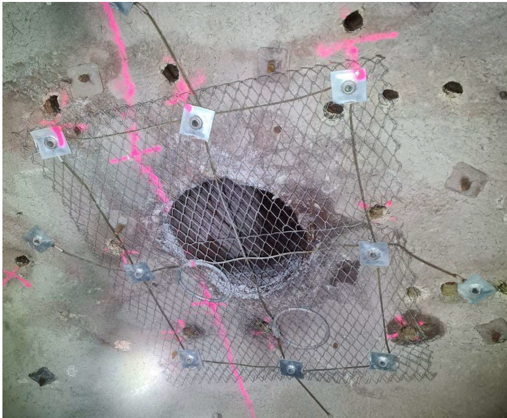
Figure 14 In situ testing of Geobrugg MINAX G65/4 mesh over a raisebore hole (Doran et al. 2023)
