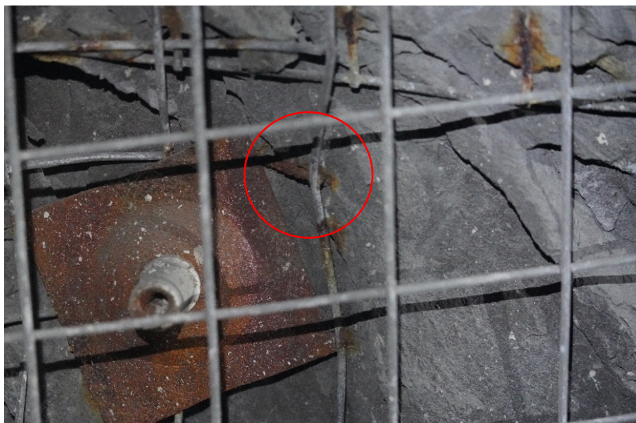
Figure 1 Observed galvanic corrosion in partner mine where metal ground support contacts the graphite-like rock
