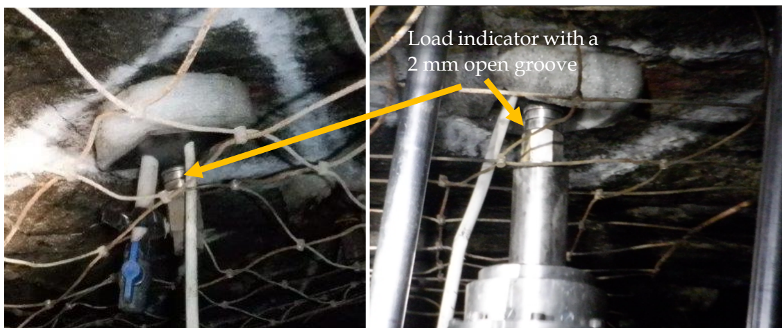
Figure 10 Uncollapsed 15 t load indicator with an open groove before pre-tension
