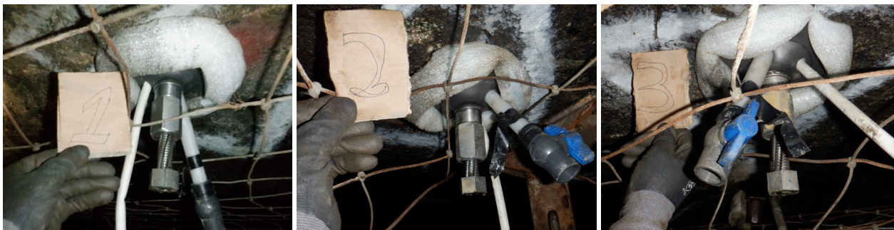
Figure 11 Collapsed 15 t load indicator after pre-tension
