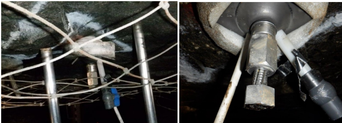
Figure 5 The 4 m long Mohlalefi dual-nut, high pre-tension cable bolts before and after tensioning with the torque multiplier
