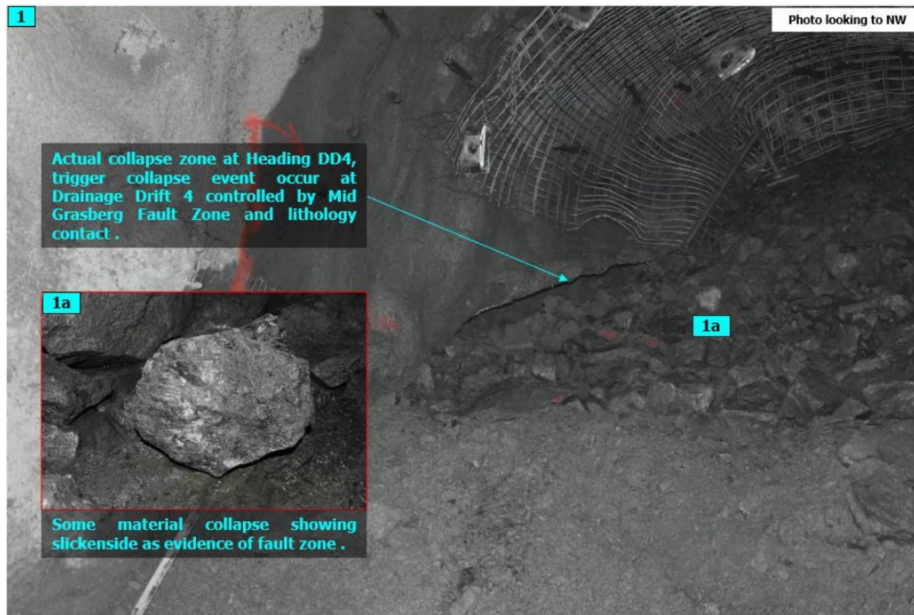
Figure 2 Ground collapse at the heading of GC2710L Drainage Drift 4 (Ekaputra 2018). The inset shows slickenside textures as evidence of the fault zone
