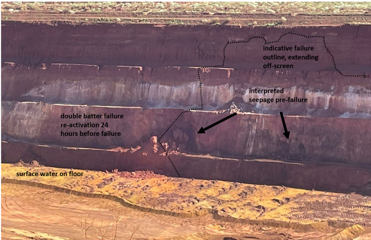
Figure 8 Failure area 24 hours pre-failure, showing reactivation of a previous double batter failure. Dark patches on walls interpreted as seepages. Surface water on pit floor inferred to be perhaps 10 cm, with some islands
