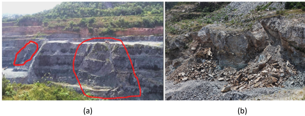
Figure 11 Pictures of instabilities influenced by major structures in (a) Zone 1 and (b) Zone 2
