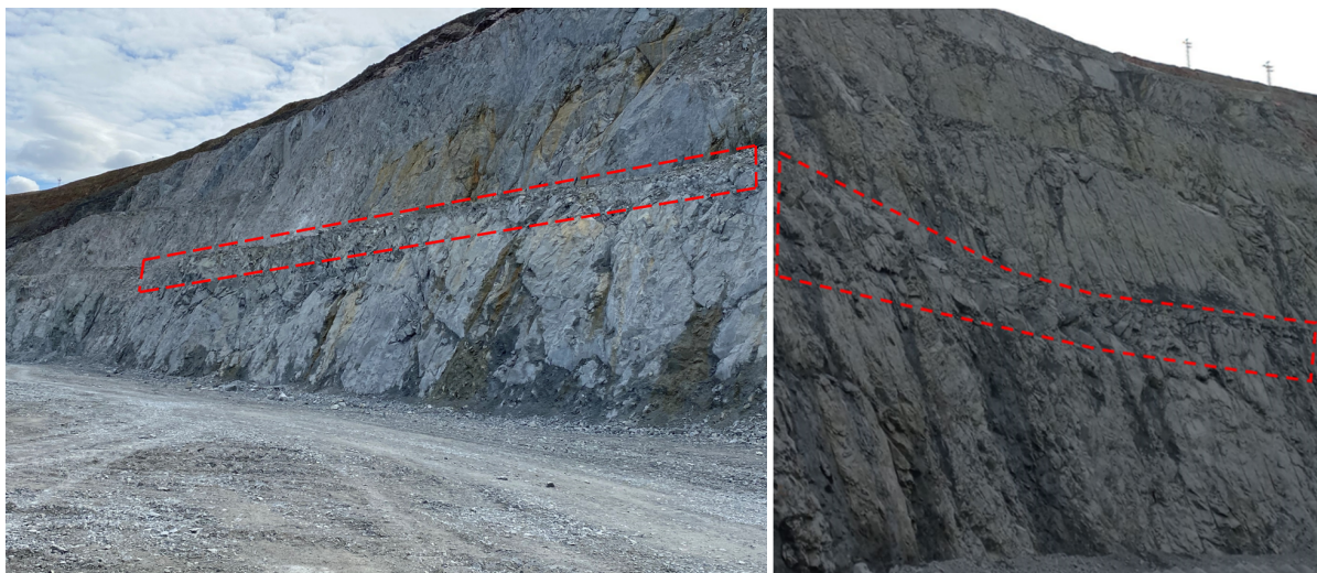
Figure 16 Crest damage due to improper sub-drilling in the proximity of the designed crest
