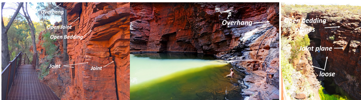
Figure 3 Google Earth-registered photograph of the rockfall risk over a walkway grating with exposed bedding and joints in Karijini National Park in the Pilbara, Western Australia
