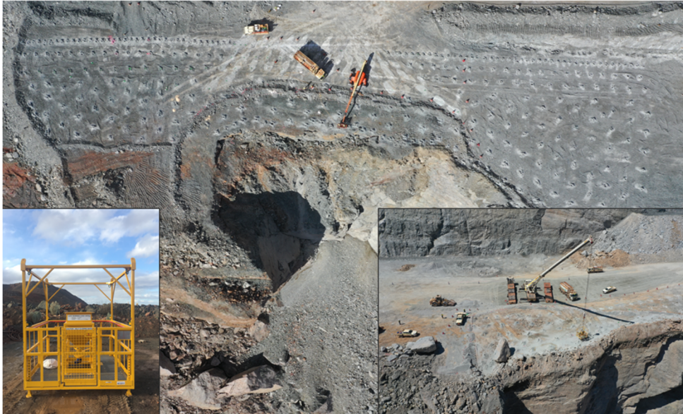
Figure 7 (Left) Image of the work cage; (Middle) The elevated work platform loading ammonium nitrate fuel oil; (Right) The work cage loading stemming within the control zone
