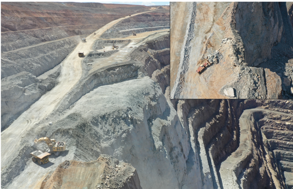
Figure 9 Image of a shovel and remote-controlled front-end loader relocating material above the East Wall Slip
