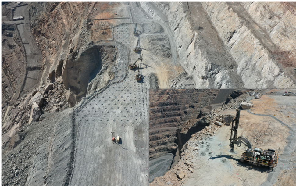
Figure 6 Probe rigs drilling holes outside of the control zone and a remote rig drilling blastholes within the control zone
