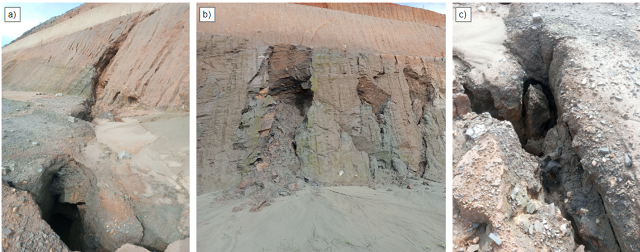
Figure 16 The effect of rainfall on the dispersive saprolites, showing piping in the slope. (a) Erosional channel through the joint; (b) Fall-out of saprolite material from the joints; (c) Erosion channel
