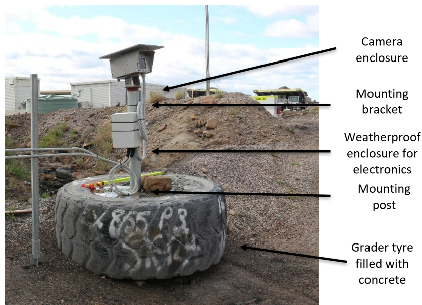
Figure 5 Picture of the whole redesigned system as installed at the mine site
