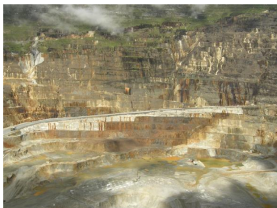
(f) Vertical crest piles, cable-dowels and mesh sprayed with fibre-reinforced shotcrete beneath mine access road located in the 60-80m thick thrust fault zone (Nov 2011)
