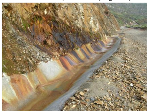
(c) Mesh and fibre-reinforced shotcrete drain; in-drain mini flow arrest dams, downslope LV access ramp, Berlin, West Wall (May 2010)
