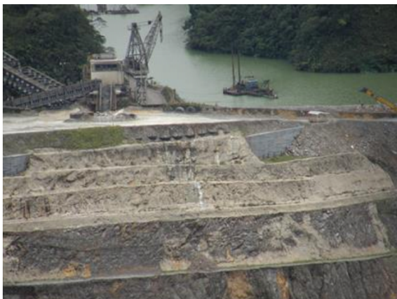
(d) Final-Slope in Photo (c); bench face beneath mine office and crusher; 1-2m thick thrust fault zone at 10-20m below reinforced slope (Feb 2007)
