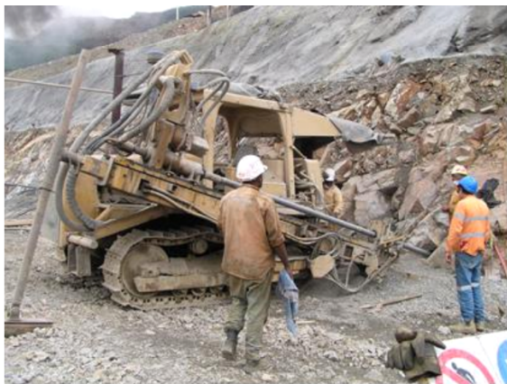
(c) Work-in-progress; meshed, 10-strand, 100t tensioned cable anchored, fibre-reinforced shotcrete sprayed bench face beneath mine office and in-pit crusher (May 2006)
