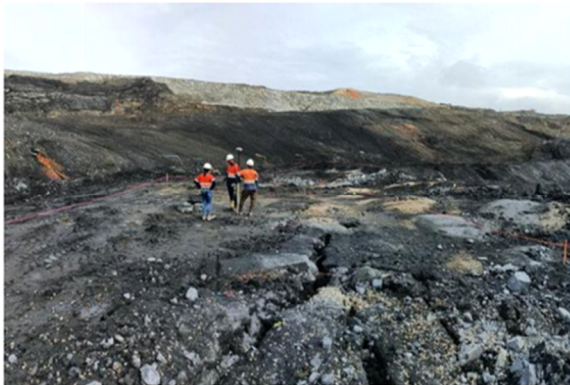
(e) significant backbreak from blasting induced gas-jacking along bedding planes; Pueblo Viejo, Dominican Republic, N slope (2021)
