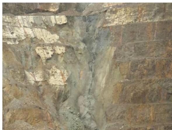
(d) Zoom of damage on ground-reinforced 15m high bench faces beneath pit haul road, with debris blockage of shafts to drainage tunnel; Ok Tedi, PNG; Berlin Chasm (Oct 2014)
