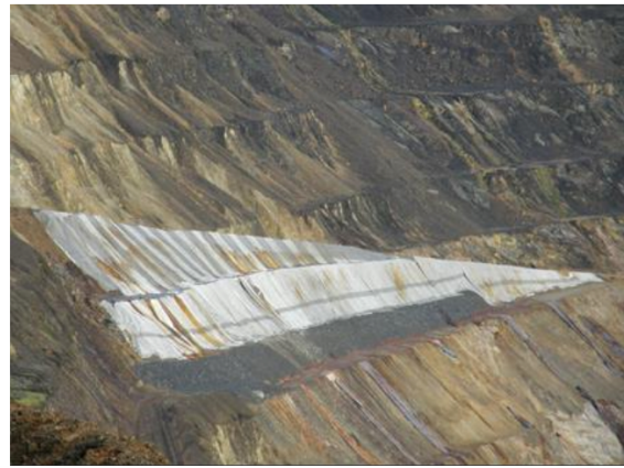
(b) Geotextile cloth covered face of access ramp to toe of Edinburgh Chasm (Jan 2008)
