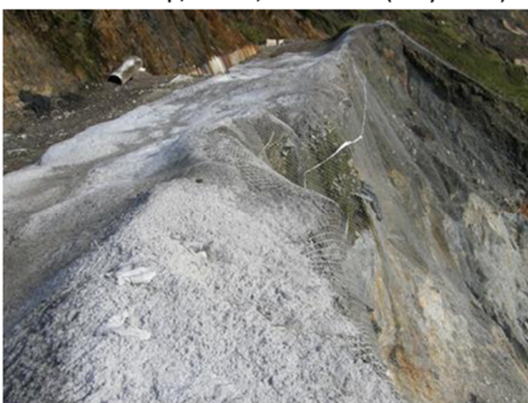
(e) Chasm crest reinforced with shear piles, mesh and fibre-reinforced shotcrete; Berlin Chasm, West Wall (Sep 2012)
