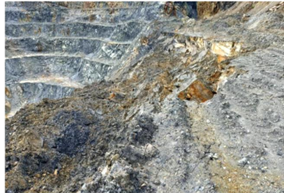
(f) Same as (e), plus unmanaged surface water flow inducing toppling instability (Pueblo Viejo, Dominican Republic, SW slope (2021))
