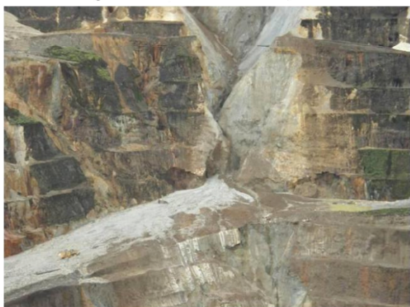
(c) Hard-attempted, but insufficient water runoff control on benches; chasm debris runoff onto haul road, cascading to pit floor below, 15m high benches; Ok Tedi, PNG (Oct 2014)
