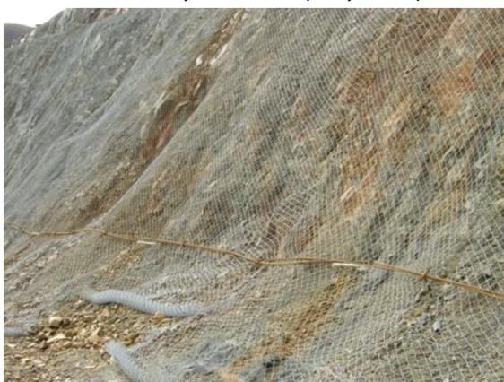
(e) Mesh, cable-dowels (before fibre-reinforced shotcrete) beneath mine access road in 60-80m thick thrust fault zone; Ok Tedi, PNG; Paris-Berlin SW slope (Apr 2012)
