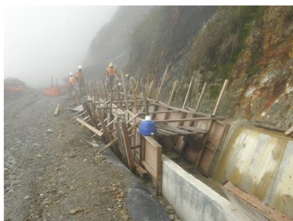
(d) Construction of cast in-situ concrete culvert open drains along downslope LV access ramp; Berlin area, West Wall (June 2011)
