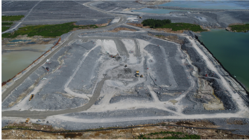
Figure 3 Construction of a massive shear key on competent foundations at Canadian Malartic Mine to remove brittle materials in the foundation.
