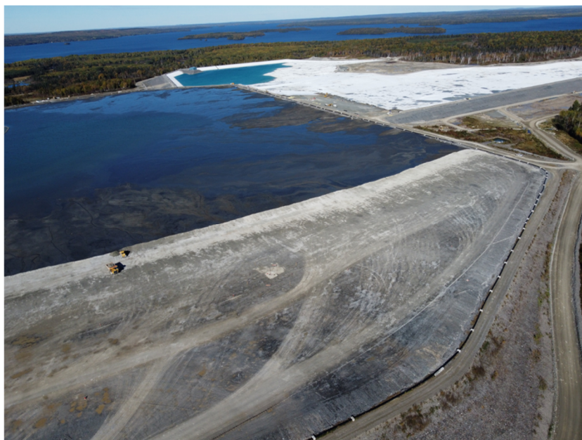
Figure 10 LaRonde Mine in Quebec (2022). An existing cell full of tailings is re-used to place filtered tailings on top of a platform (bridge lift) of rockfill (2.0 m). This figure shows a partial bridge lift.
