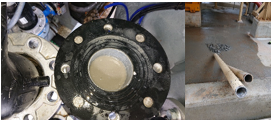
Figure 8 Initial challenges with the binder slurry plant; examples of cement blockages
