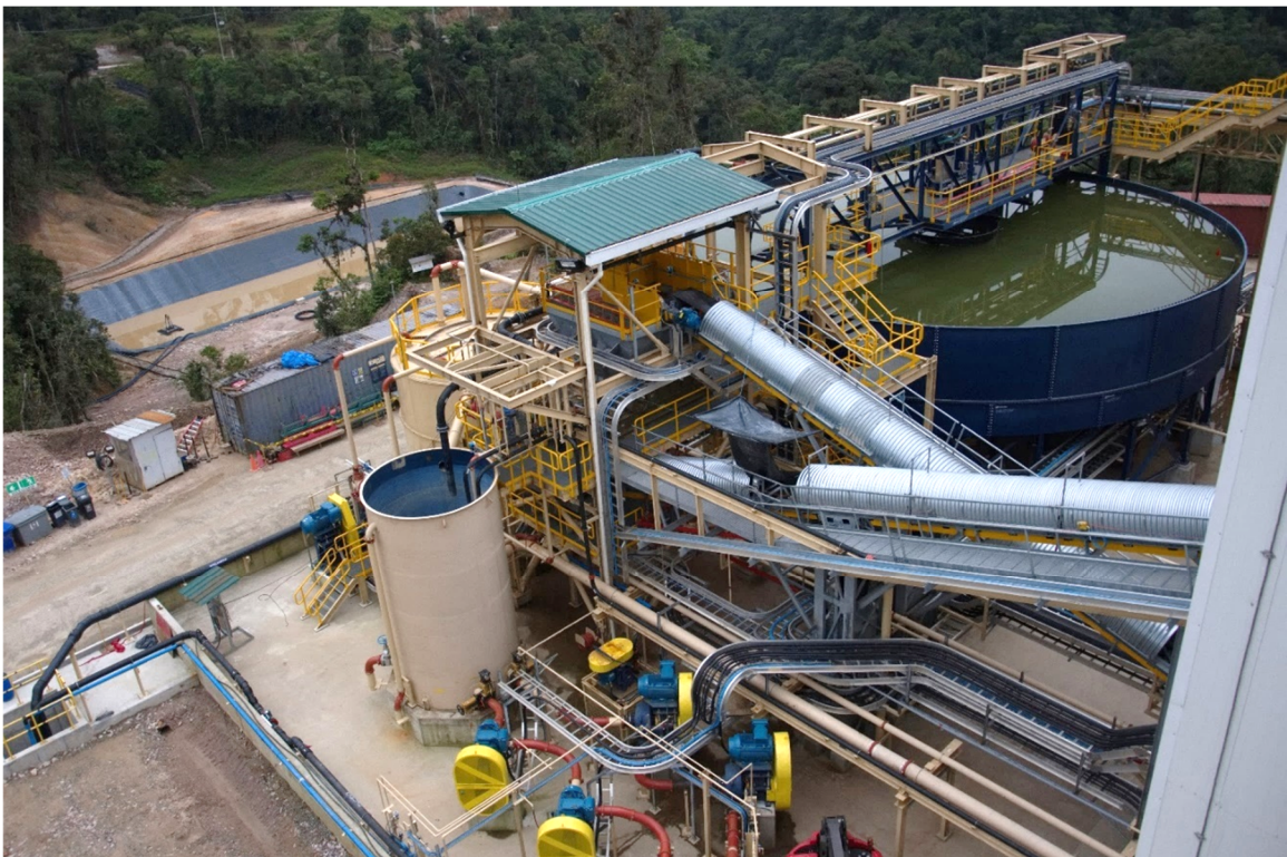
Figure 10 Tailings feeder with switchback conveyor arrangement
