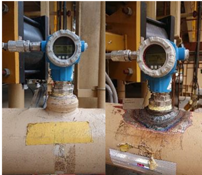
Figure 14 Flush mounting instrumentation to eliminate cemented blockages
