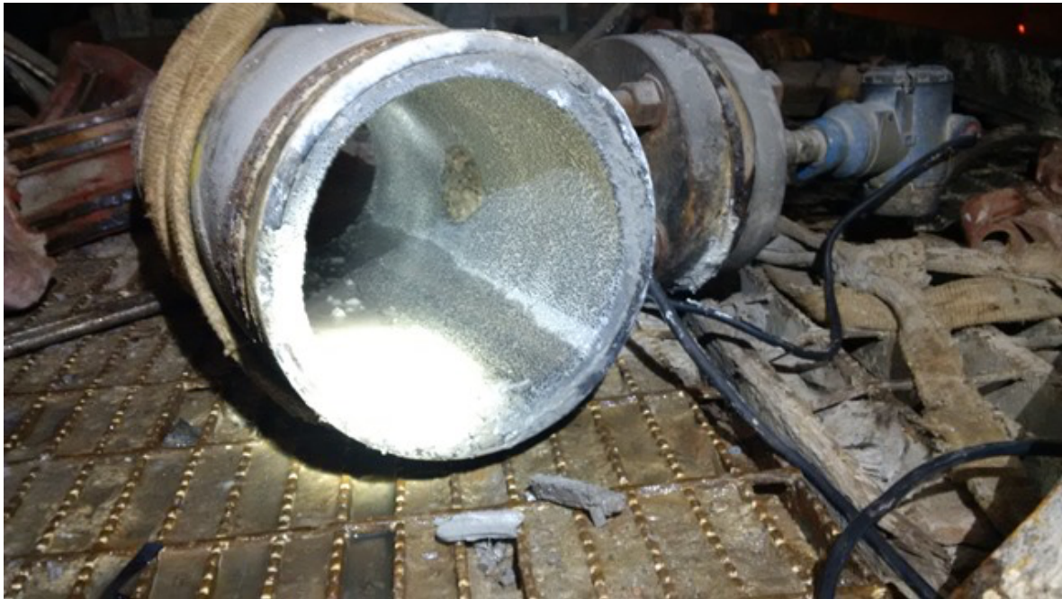
Figure 1 Dead leg of pressure transmitter branch filled with cemented paste
