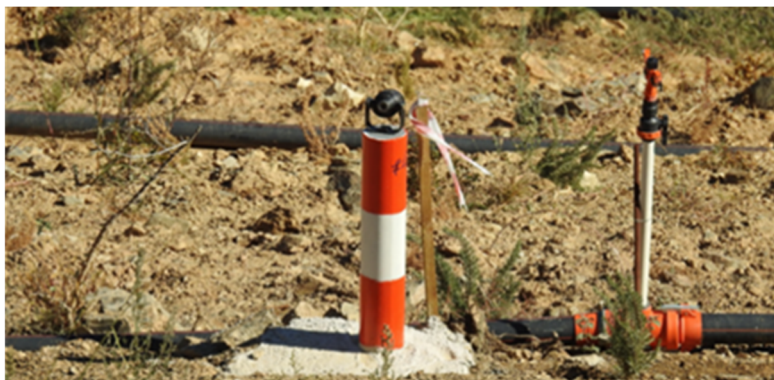
Figure 18 Survey prism station for monitoring deformation and settlement
