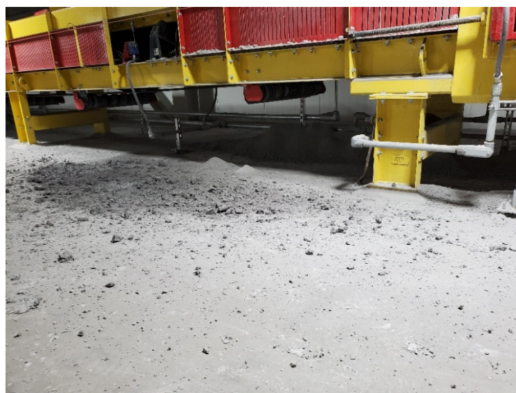
Figure 12 Filter cake spillage at take-away conveyor loading point after three filter cycles
