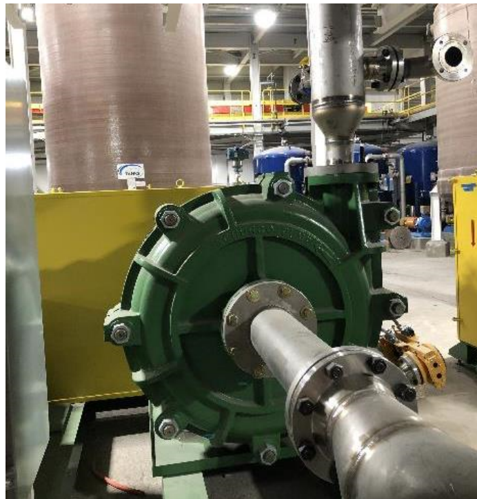
Figure 7 One of three installed filter feed pumps
