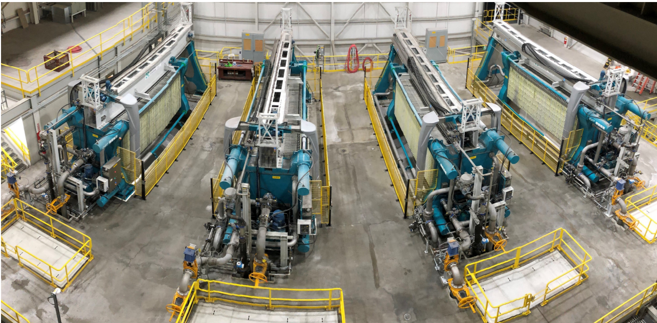
Figure 8 Four installed Aqseptence GHT2000.p7 recessed chamber pressure filters
