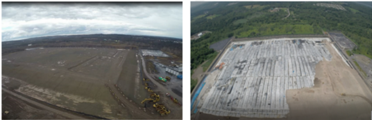
Figure 8 Example of reclamation of geotextile tube deposits after capping (adapted from TenCate Geosynthetic Americas).
