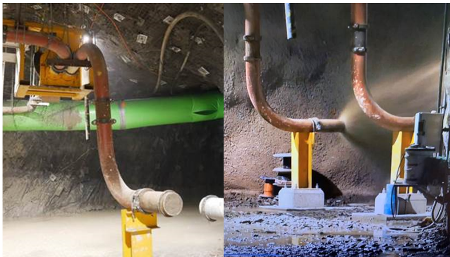
Figure 14 Photographs showing the blocked choke station piping and clearing those pipes
