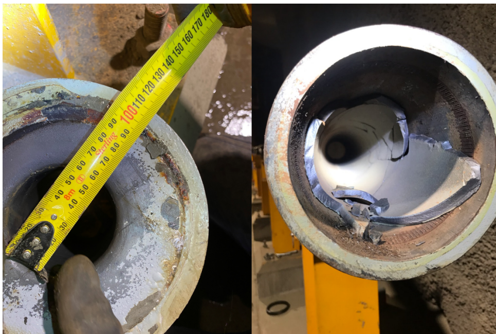
Figure 12 Two photographs showing the appearance of a choke during a routine wear inspection (RHS) and the ceramic in one of the spacers after installation
