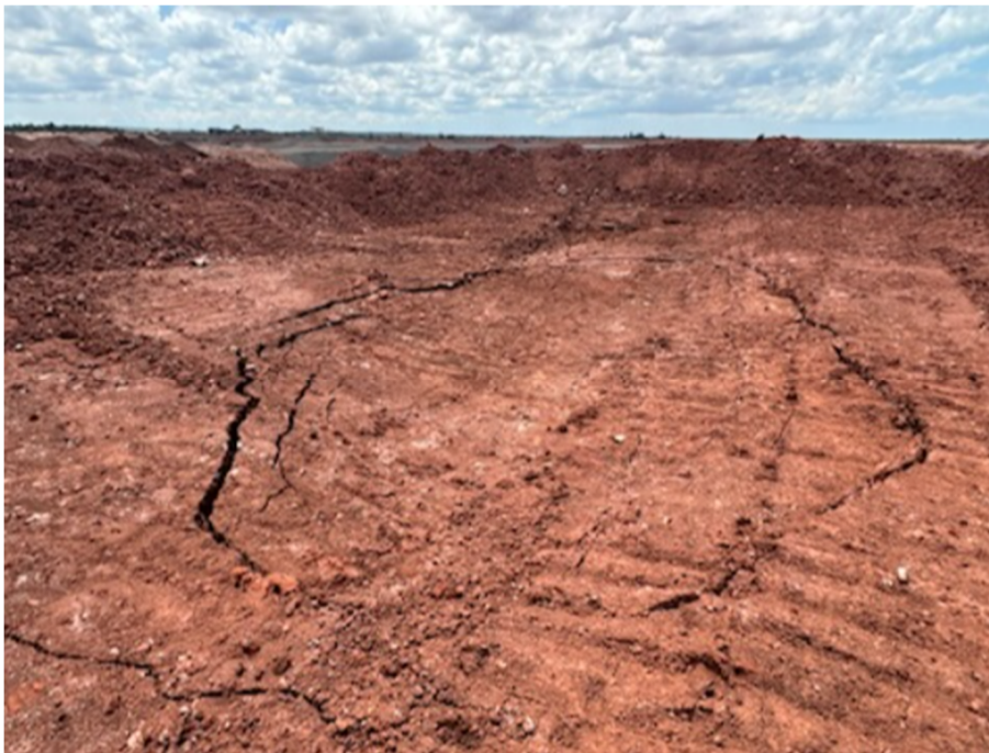
Figure 2 Localised collapse-settlement in the cover 'reshaping fill' after the first rainy season
