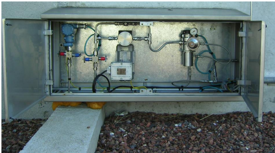
Figure 6 Measuring apparatus installed at the head of a pressure-relief borehole to continuously monitor the barometric pressure, the wellhead pressure (i.e. mine reservoir pressure) and the methane content of the mine gas (photography by French Department for Mine Safety and Risk Prevention)
