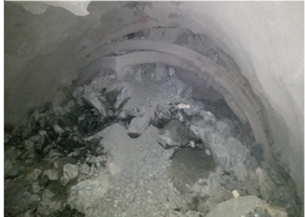
Figure 2 Typical failure of bottom infrastructure roadways at Lift 530 m.
