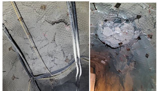
Figure 4 Instances of heavily damaged yet contained ground support following Strainbursts in Block Caving Operations.
