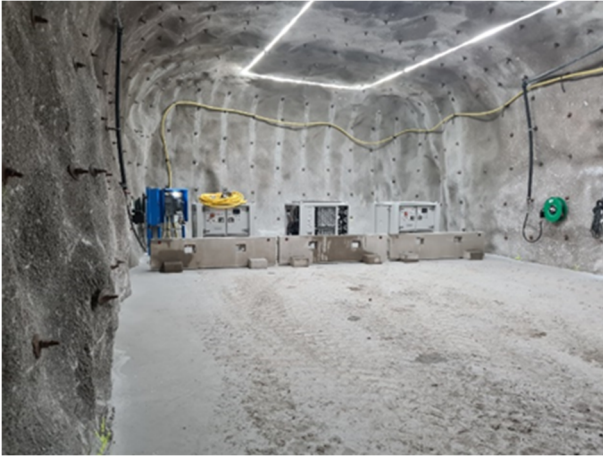
Figure 4 Level 1232 charging bay with two chargers and a cooler.
