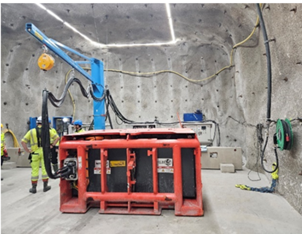
Figure 5 Charging bay with swing arm installed.
