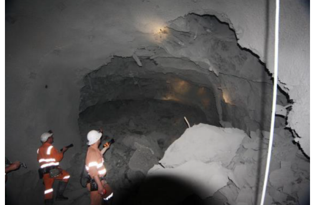
Figure 8 RWD undercut drive after September seismic event showing scarp of Red Fault and splay in foreground.
