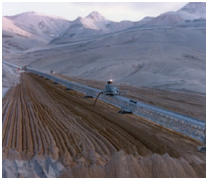
Figure 1 The Rako filter stack tailings storage facility at the La Coipa mine (Vargas & Campomanes 2022)
