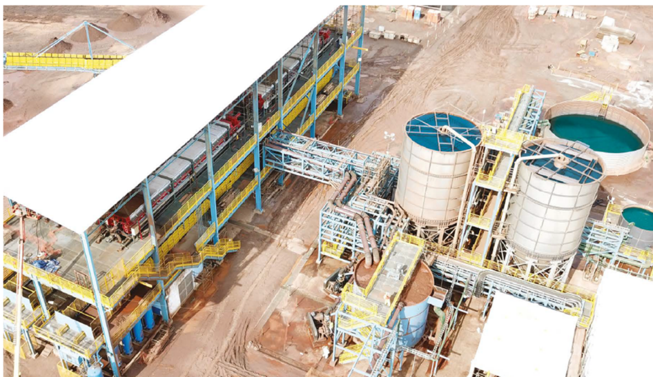
Figure 7 Matec filtration plant in Brazil 2019
