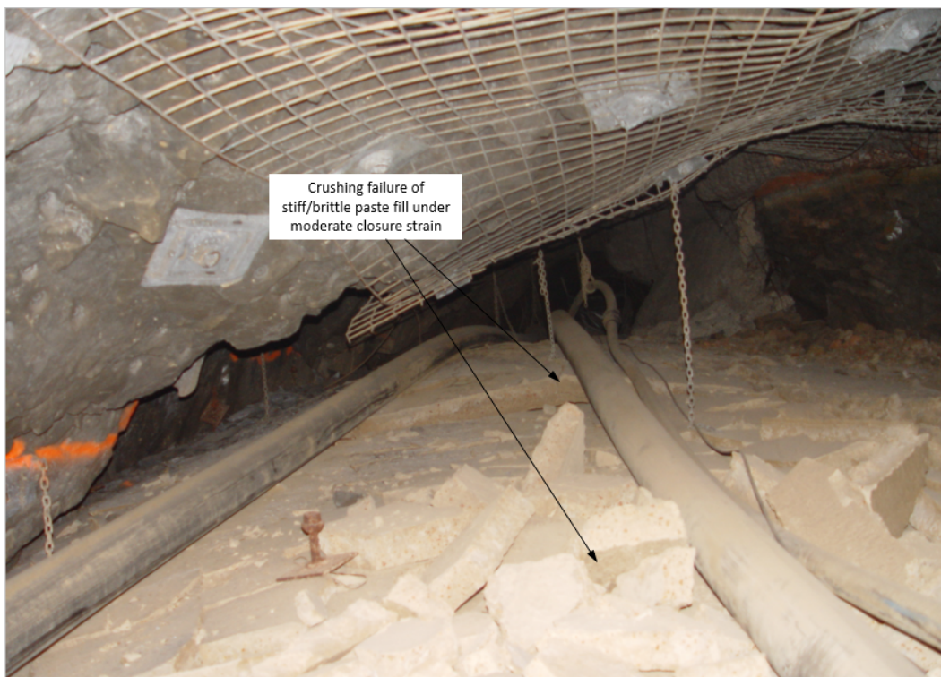
Figure 3 Example of damage to stiff cemented paste backfill due to moderate drive closure
