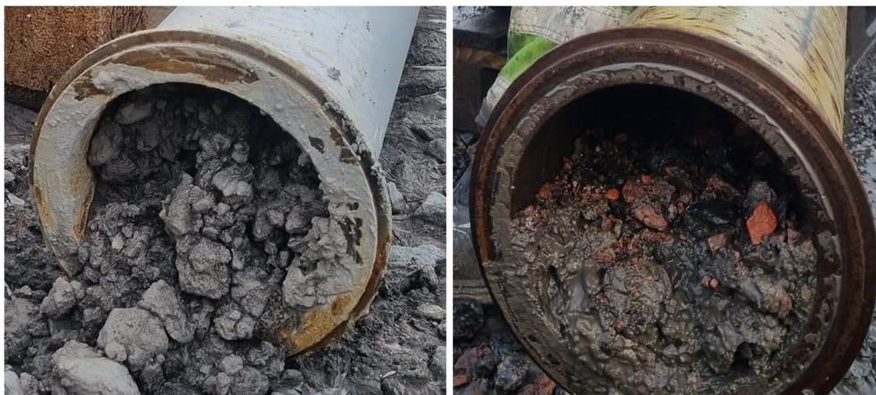
Figure 4 Blockage in pipelines
