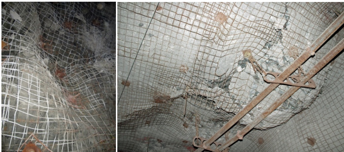
Figure 31 Ground support systems (domed plates, welded mesh, and mesh straps) containing a rockburst (Simser 2018)
