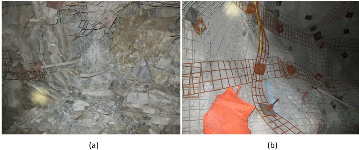
Figure 30 (a) Failure of mesh around the plate (left bolts) and failure of the bolt head at the plate (right bolt), illustrating surface support/connection failure; (b) Poorly installed mesh strap
