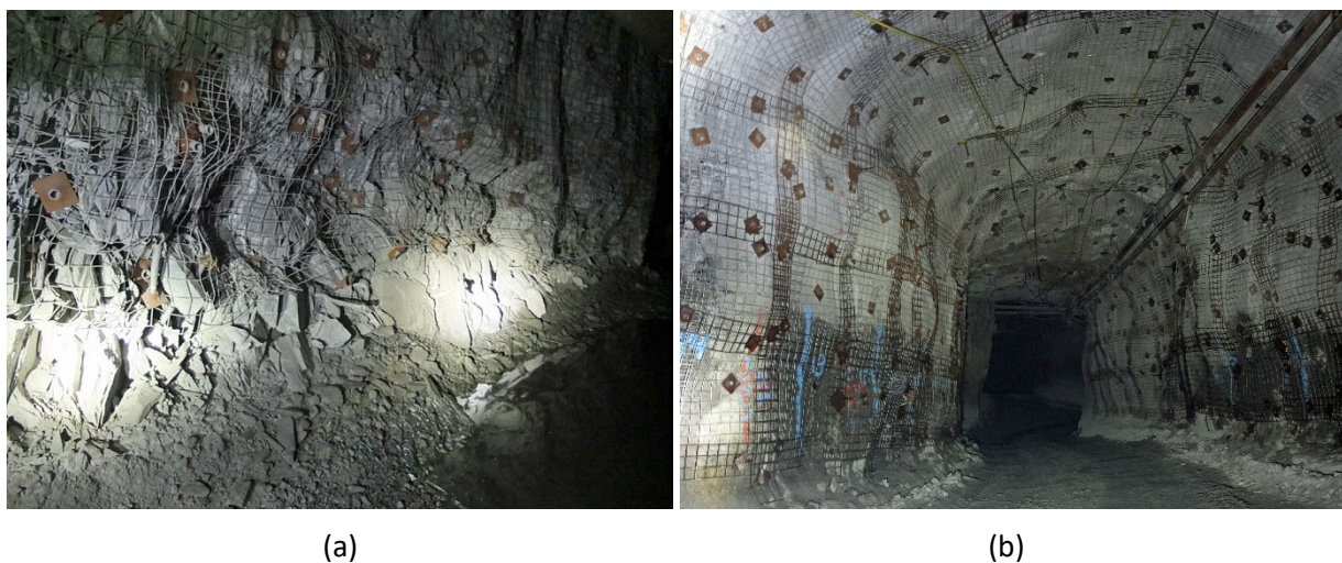
Figure 38 (a) Deterioration associated with lack of support to the floor; (b) Ground support installed to the floor
