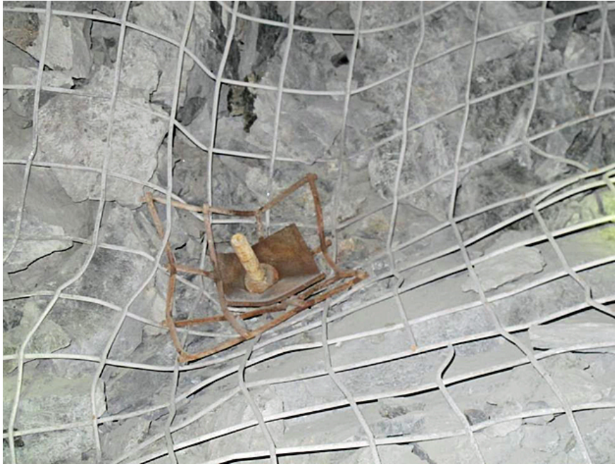
Figure 32 Paddled energy-absorbing rockbolt with collapsed dome plate over top of deformed wire mesh strap plate (Simser 2019)
