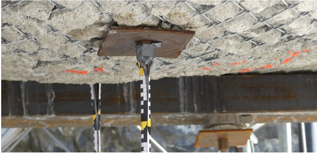
Figure 12 Post-test MINAX 80/4.6 central bolt detail
