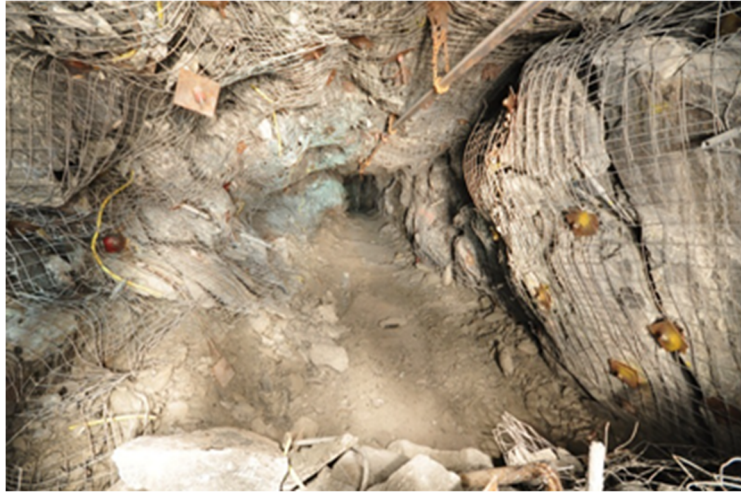
Figure 1 Significant damage to ground support and excessive deformation at Lapa gold mine
