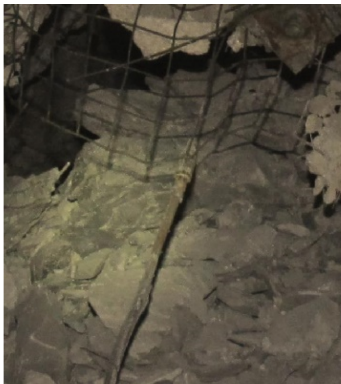
Figure 8 Seismic event occurred on 3 October 2018, at F7775NOD, showing Garford bolt yielded to the limit of its capacity
