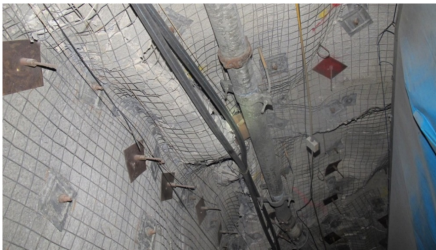
Figure 6 Seismic event occurred on 3 October 2018, at F7775NOD, showing loaded cable and Garford bolts
