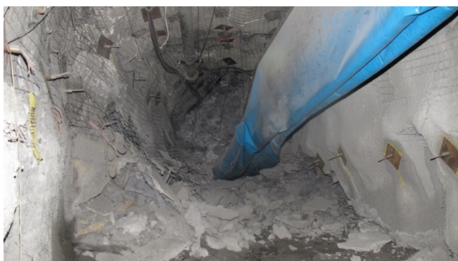
Figure 3 Seismic event occurred on 3 October 2018, at F7775NOD. Failure depth estimated at 1.5 m
