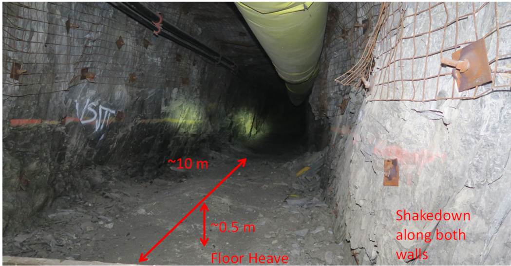
Figure 1 Photo showing floorburst damage
