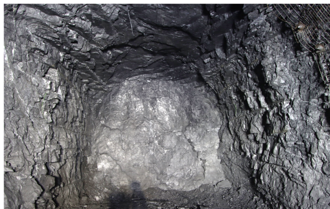
Figure 5 Crosscut face at X925 level, 25 m below the sill and looking east towards the hanging wall. Visible horizontal stress-induced fracturing is in the back. Heading width is 5.8 m and height is 5.0 m. Sub-vertical graphite surfaces are visible on the face, typical to the mineralisation
