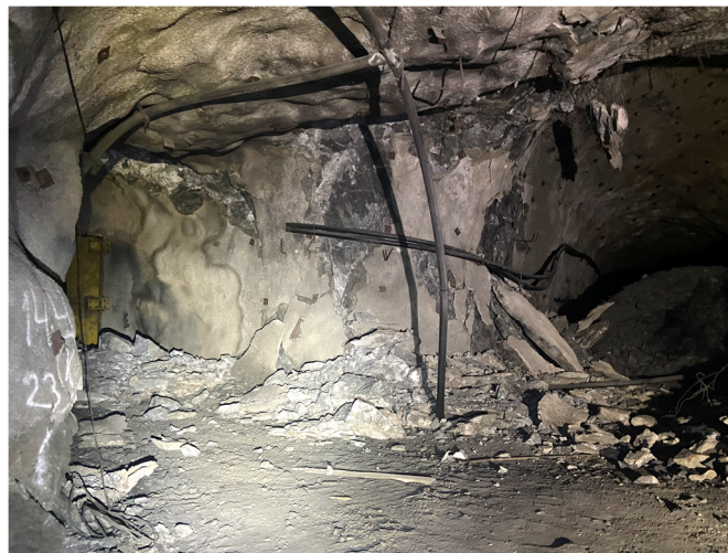
Figure 20 Damages after the event in the intersection area of the footwall drive and exhaust air raise access, looking northwest
