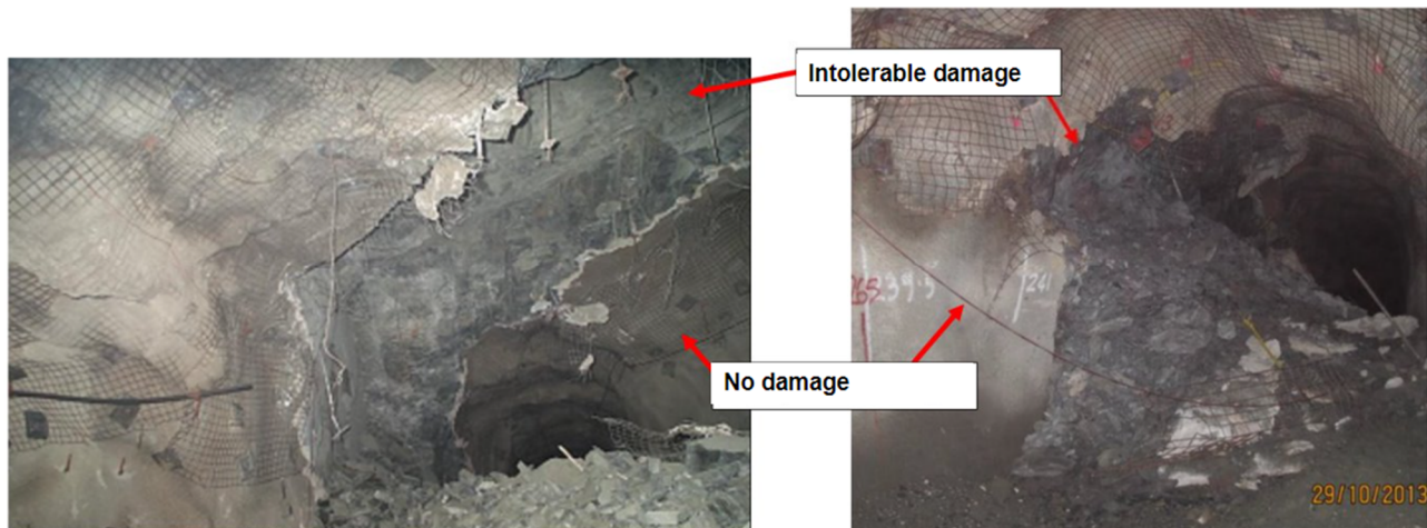
Figure 1 Photographs of rockburst damage showing the variation from no damage to intolerable damage (total destruction) of ground support within a very short distance. Note that the calculations for ground support capacity and demand would be the same for the no damage and total destruction areas
