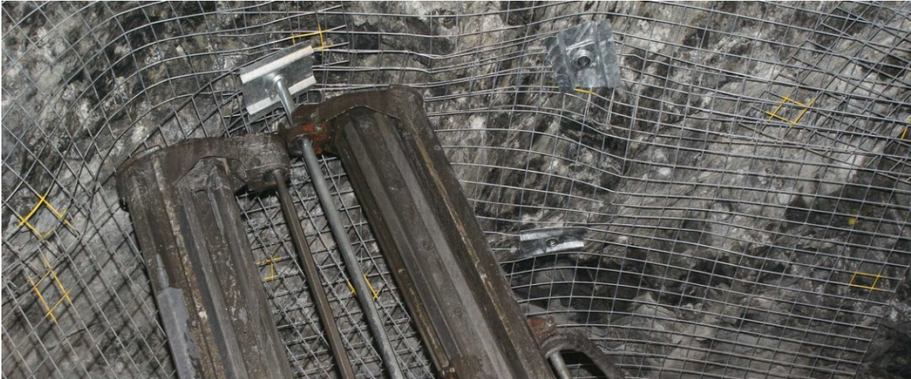
Figure 1 Installation of a mechanical hybrid rockbolt with a twin boom drill rig
