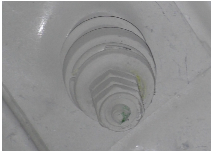
Figure 13 MD peg bolt still visible covered in blasting dust
