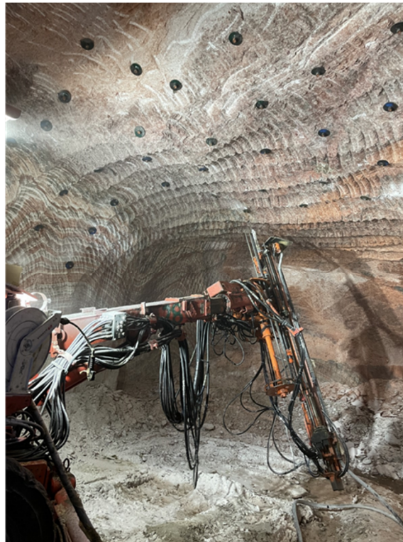
Figure 11 Installation of roof rockbolts with FASLOC SF resin cartridges at the production area
