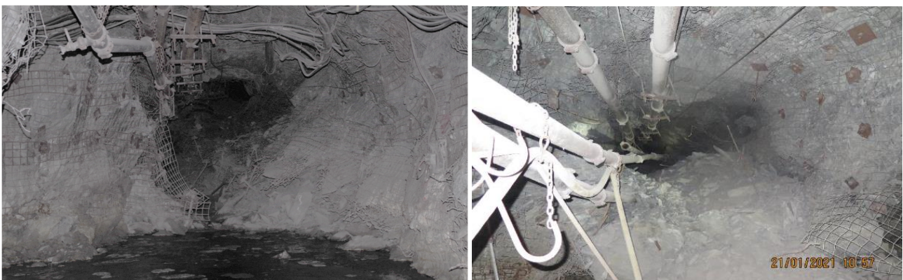
Figure 8 Example of the underground damage caused by the seismic event on 132-04 TBW (looking west) most of the visible damage came from the wall
