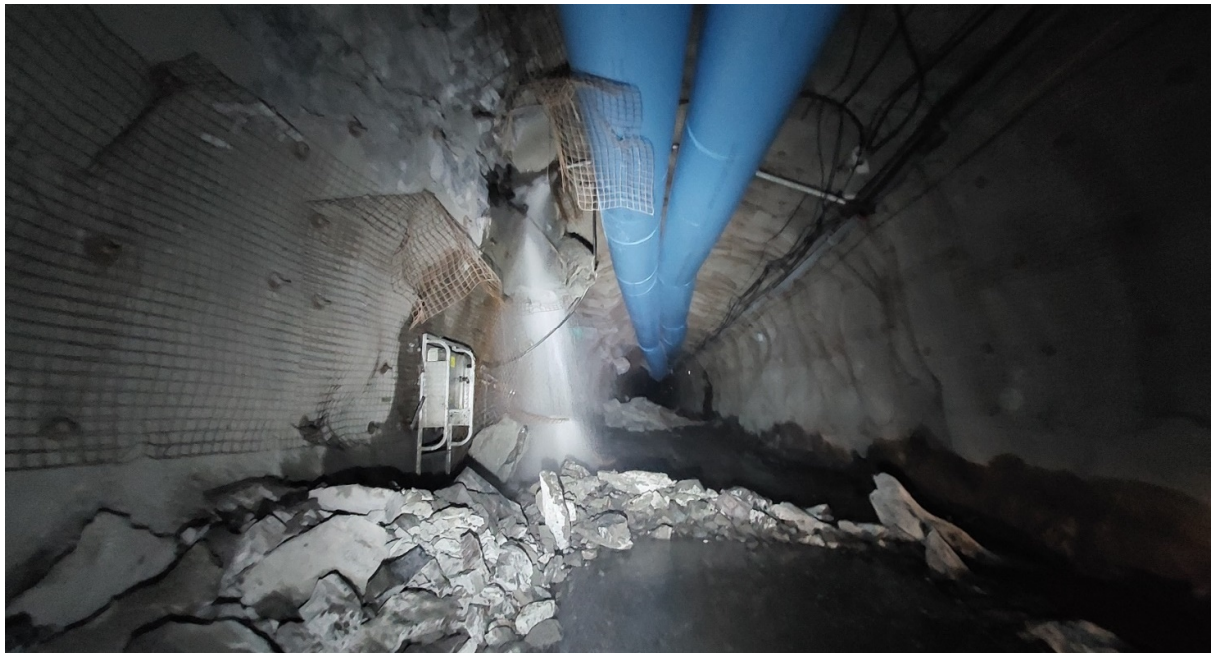
Figure 14 View of the damage from the event after some rock had been removed, looking south
