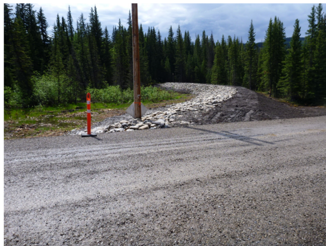
Figure 8 Diversion berm upstream of Panther Road
