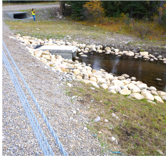
Figure 7 Inlet to low-flow culvert below Panther Road that maintains primary channel and fish spawning habitat, with inlet of high-flow diversion culvert in background
