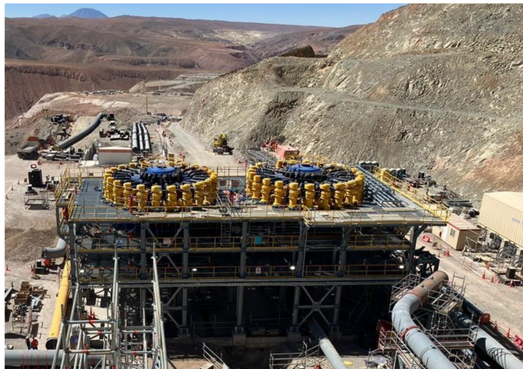
Figure 4 Cavex DE cyclone cluster for a large mining operation in Chile (courtesy of Weir Minerals)
