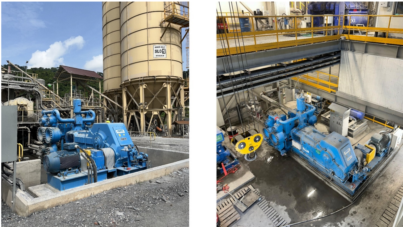
Figure 1 Medium size piston-diaphragm pumps examples in cemented paste fill plants
