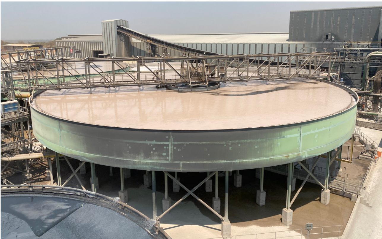
Figure 2 Kakula Phase 1 thickener in operation
