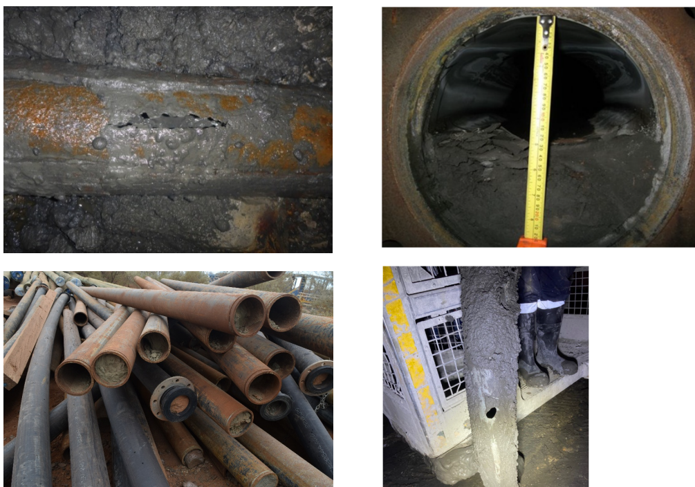
Figure 3 Examples of reticulation failures and pipe blockages
