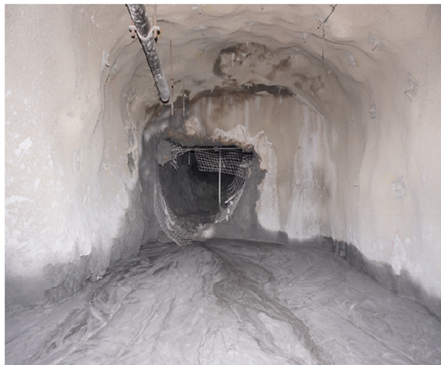
Figure 1 Example of shotcrete paste wall failure during tight filling (Gray 2019)
