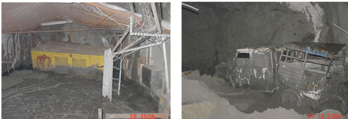
Figure 2 Examples of paste wall failure consequences (Yumlu 2007)
